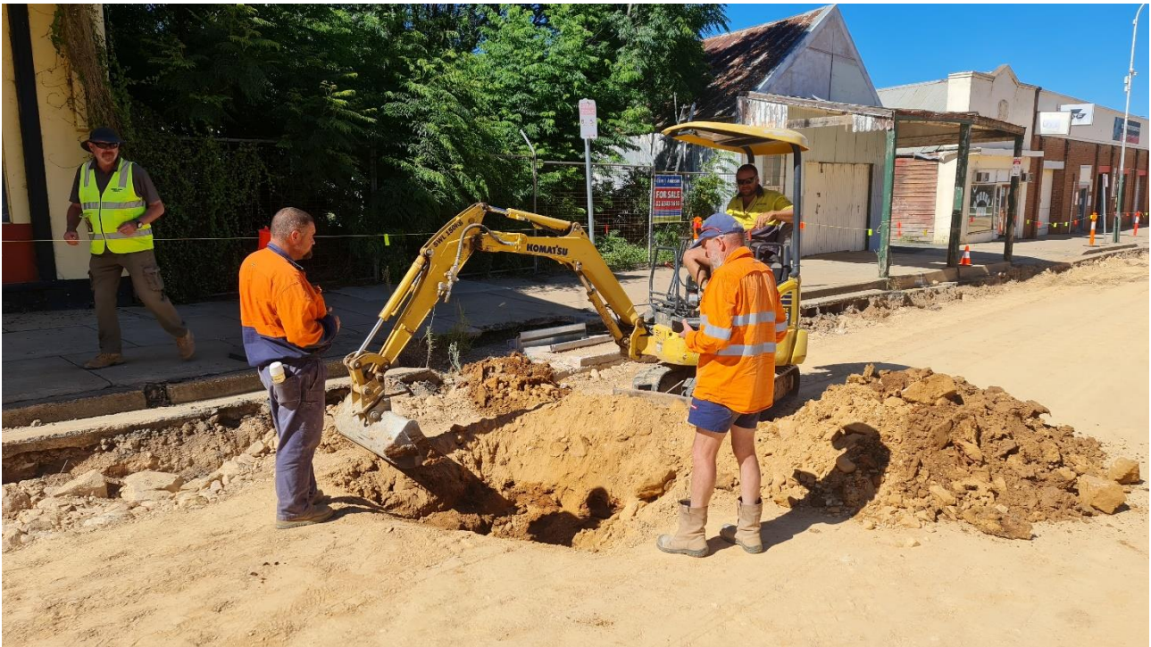
Geotechnical technician requested test pit to observe ground conditions below bridging layer
