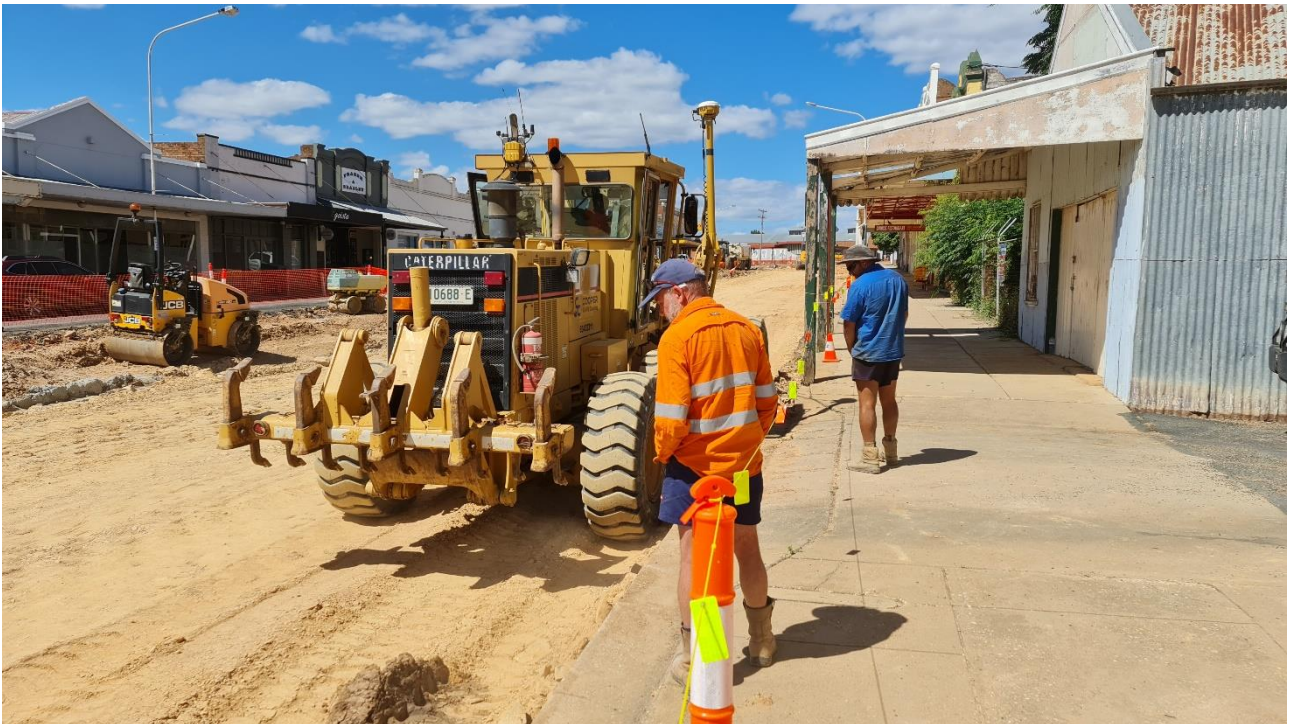
Geotechnical technician completing a proof roll test on subgrade layer, test failed...
