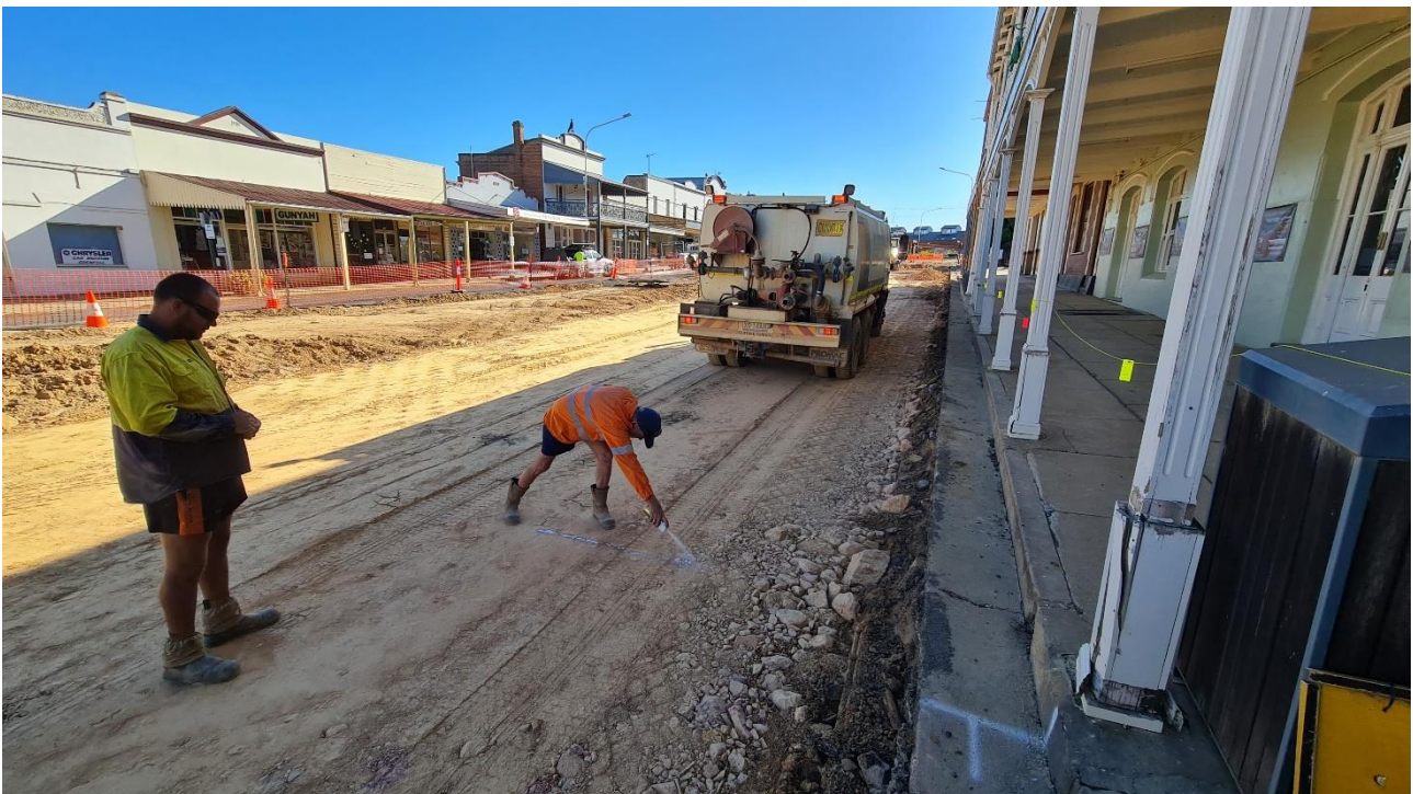
Geotechnical technician marking out locations that failed proof roll test
