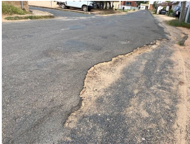
Figure 2 The George Street Road surface is very rough.
