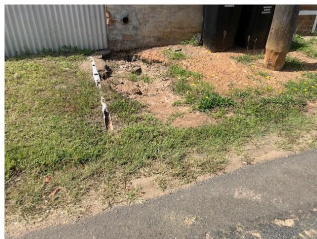
Figure 4 George Street has many trip hazards including storm water pipes.
