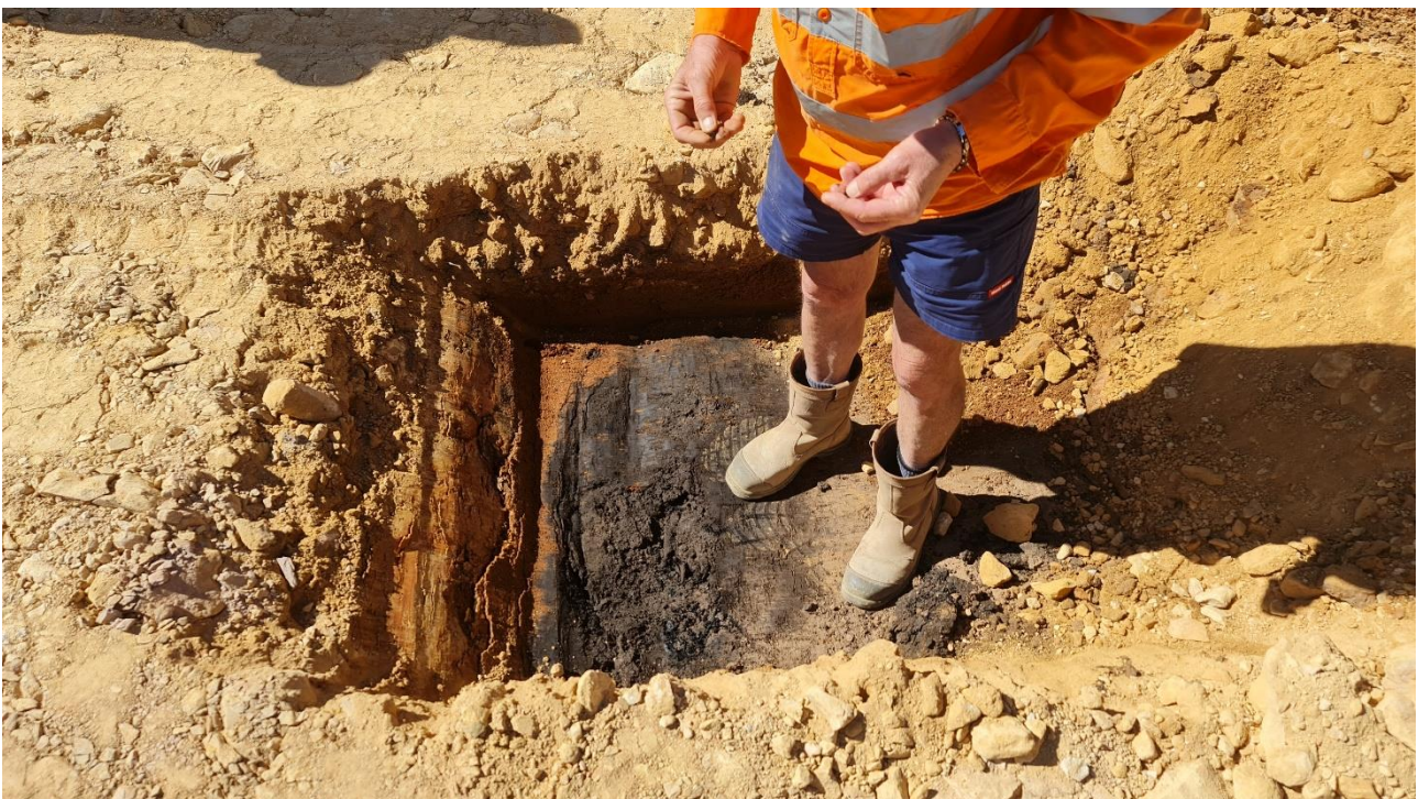
Geotechnical technician advised material under bridging layer unsuitable, additional Geotech advice sought
